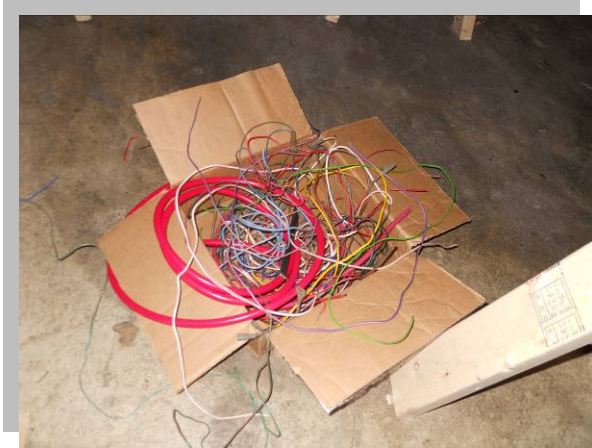
Left-over wires – anyone need some????
