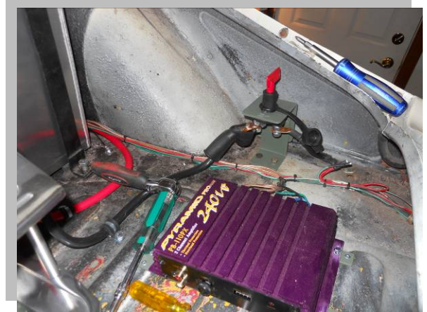
Amp and cut-off switch in the trunk...
