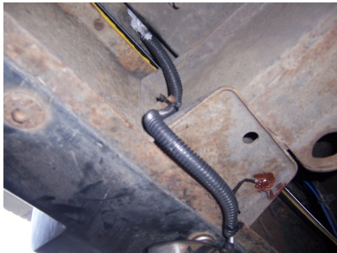
Wiring for the light – protected wire run
