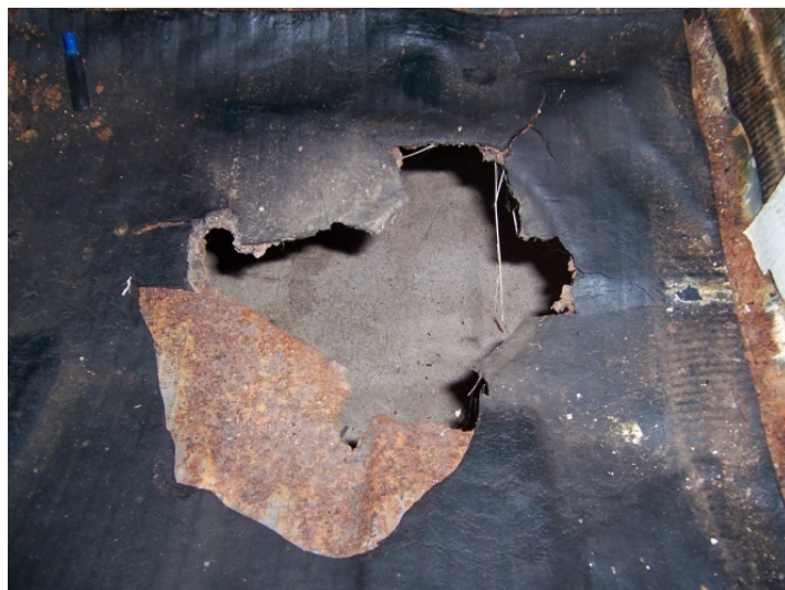
Ample evidence Rust-Proofing didn't work!
