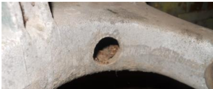
Hole in trailing arm
