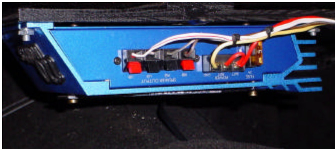
Amp in place under the battery box.
